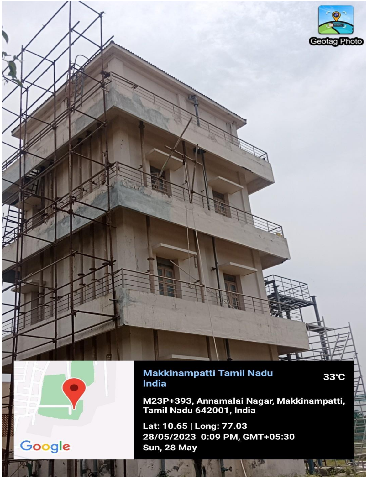
Overhead Tank constructed by MCET located in MCET playground (Capacity: 100000 liter)
