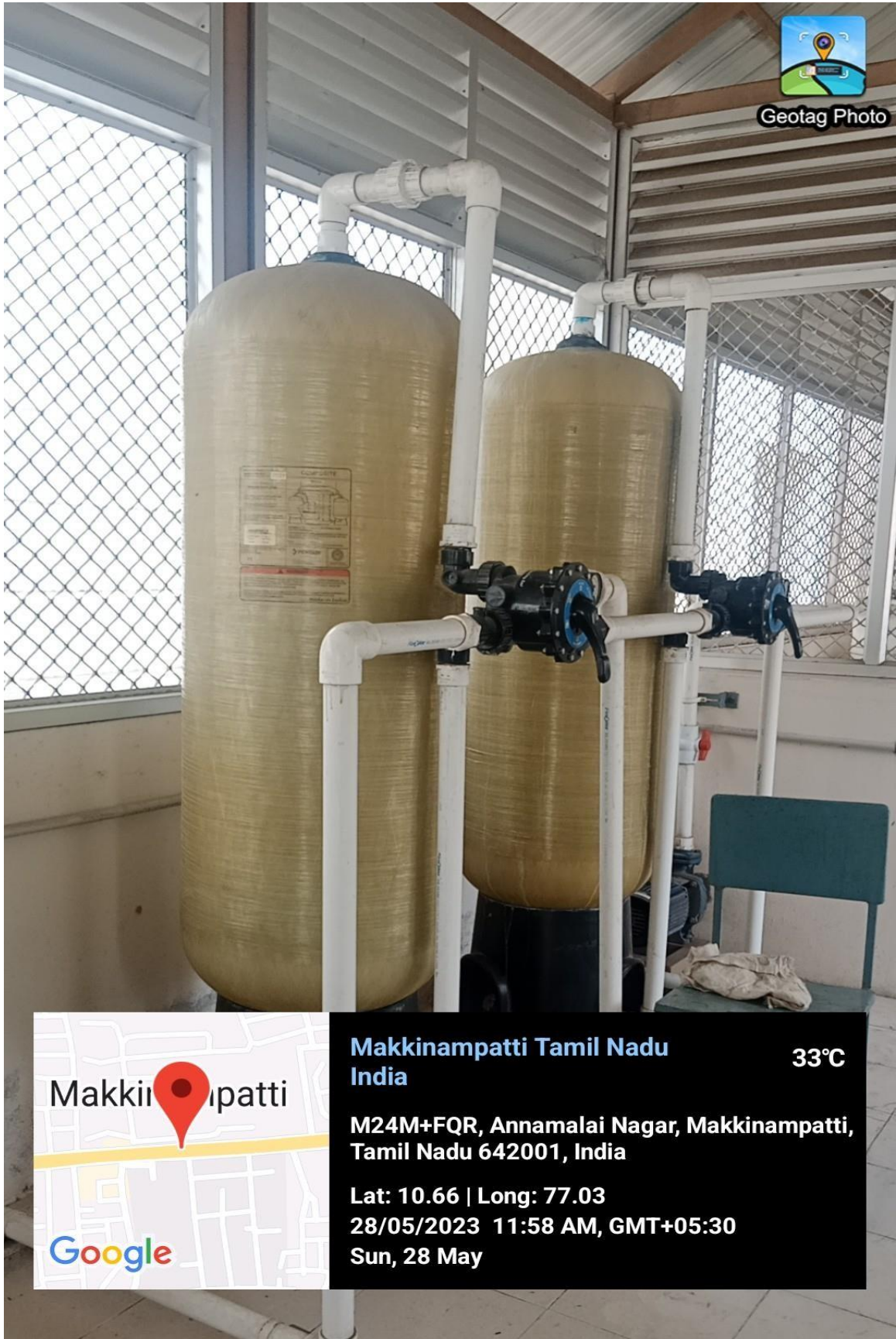
RO plant unit for filtering the water
