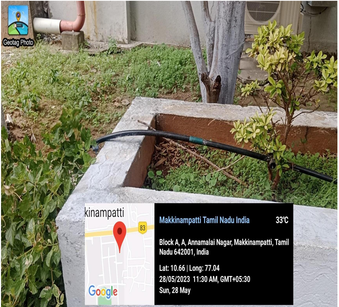
Water distribution for gardening purpose
