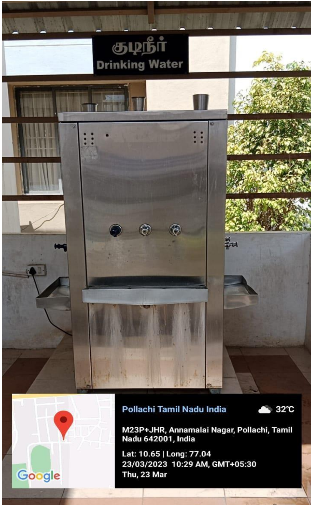
Purified water unit to distribute the water for drinking purposes
