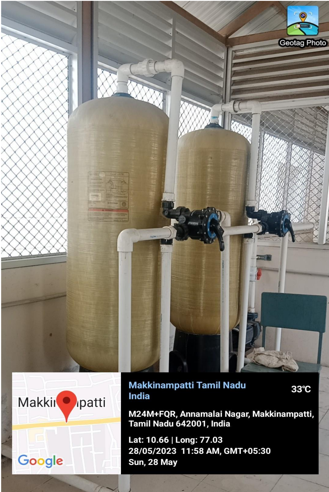
RO plant unit for filtering the water
