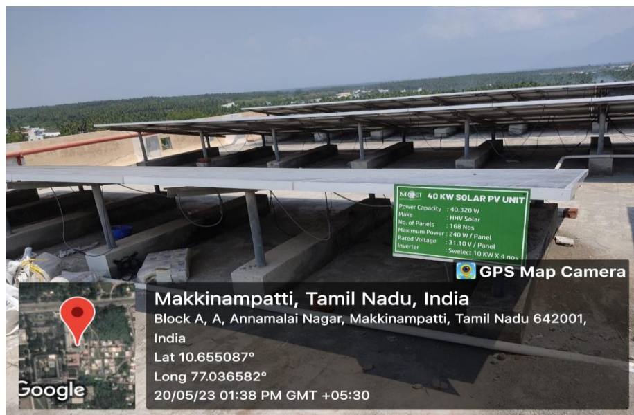
Fig.1.3 40 KW SOLAR PV UNIT
