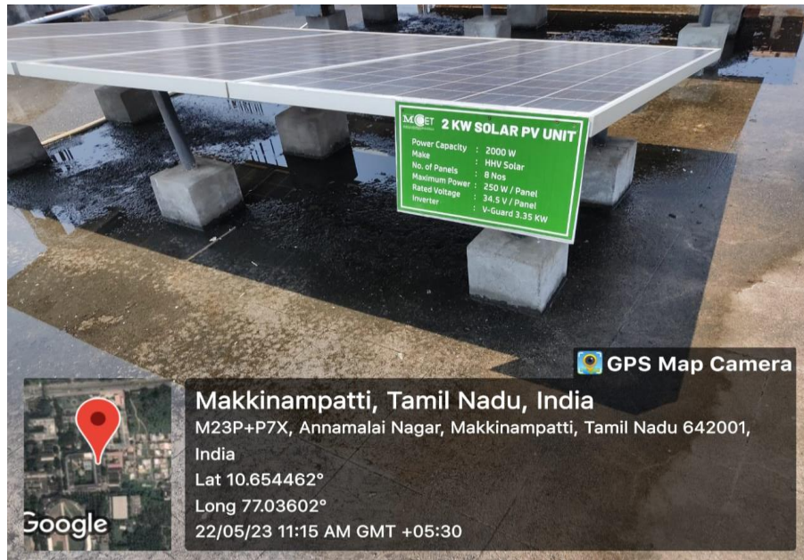
Fig.1.2 2 KW SOLAR PV UNIT
