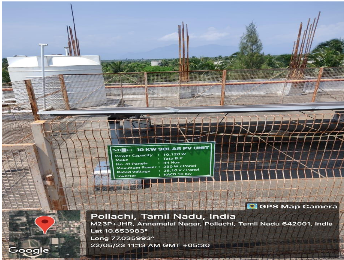
Fig.1.1 10 KW SOLAR PV UNIT
